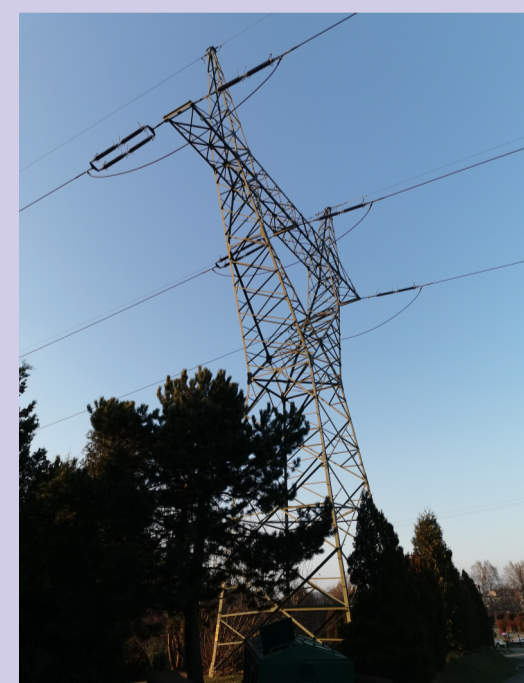
Fig. 3 Place of measurement – 100 kV power line.
